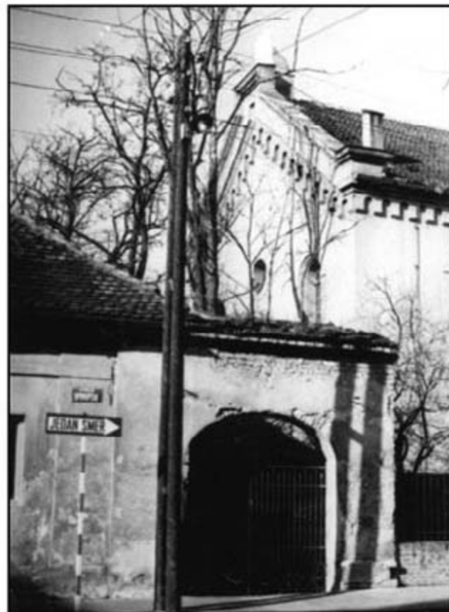
A view of the current state of the gate to the schoolyard and synagogue
