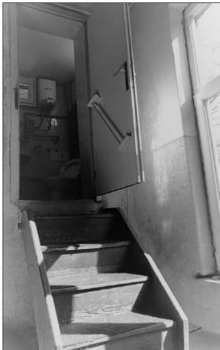
41. The elderly members can barely manage to reach the toilet from the ground floor; and, what is more, they have to use make-shift wood stairs!
